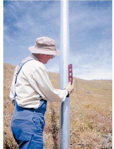
Above: Checking the tower for plumb. The turbine will only yaw properly on a plumb tower.
