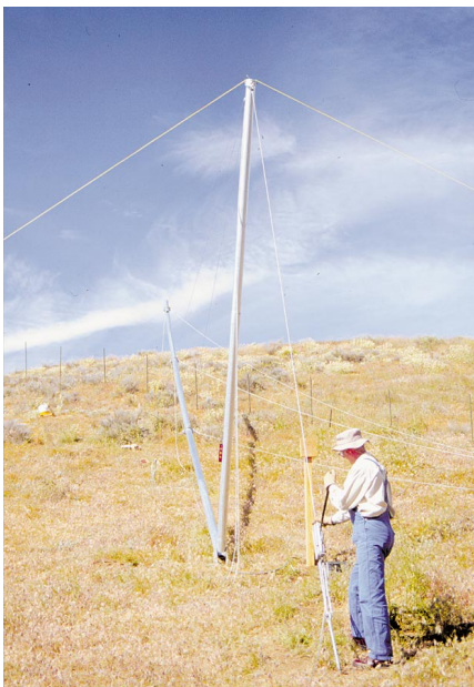
Below: The tower almost down. The forward lever on the griphoist is used to pay out cable.
