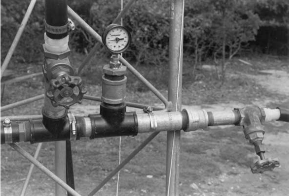
Figure 8: Pressure gague and fitting at base of test tower
