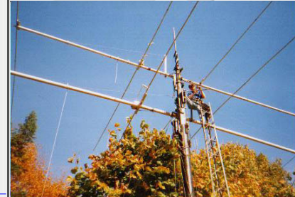
THE BIG TOWER NESTED ST 28 FT...MY SON MICHAEL WORKING FROM THE WORK TOWER, CHANGING ONE OF THE OMEGA MATCHES
