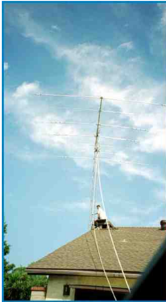
The Assembly is almost vertical now. Damon is getting ready to nest the tower into a roof eave bracket we made to hold it in place.
