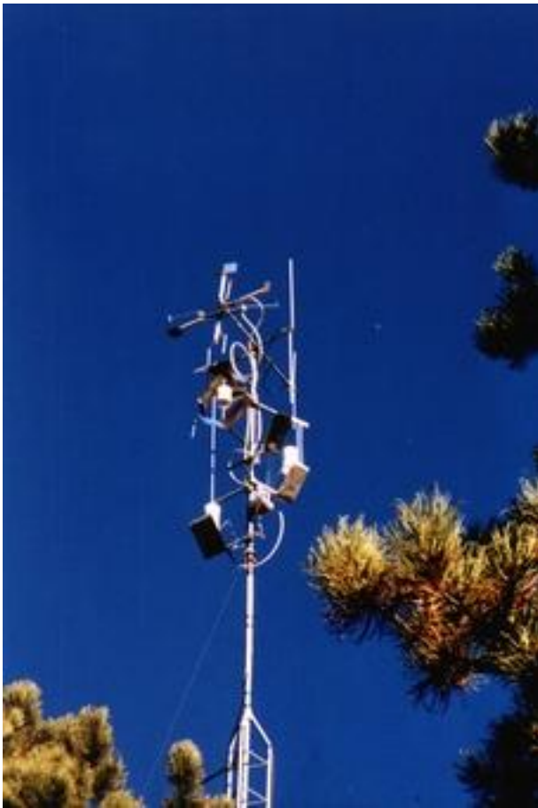
Installation at WDOEJA Multiple Isotrons on one mast!
