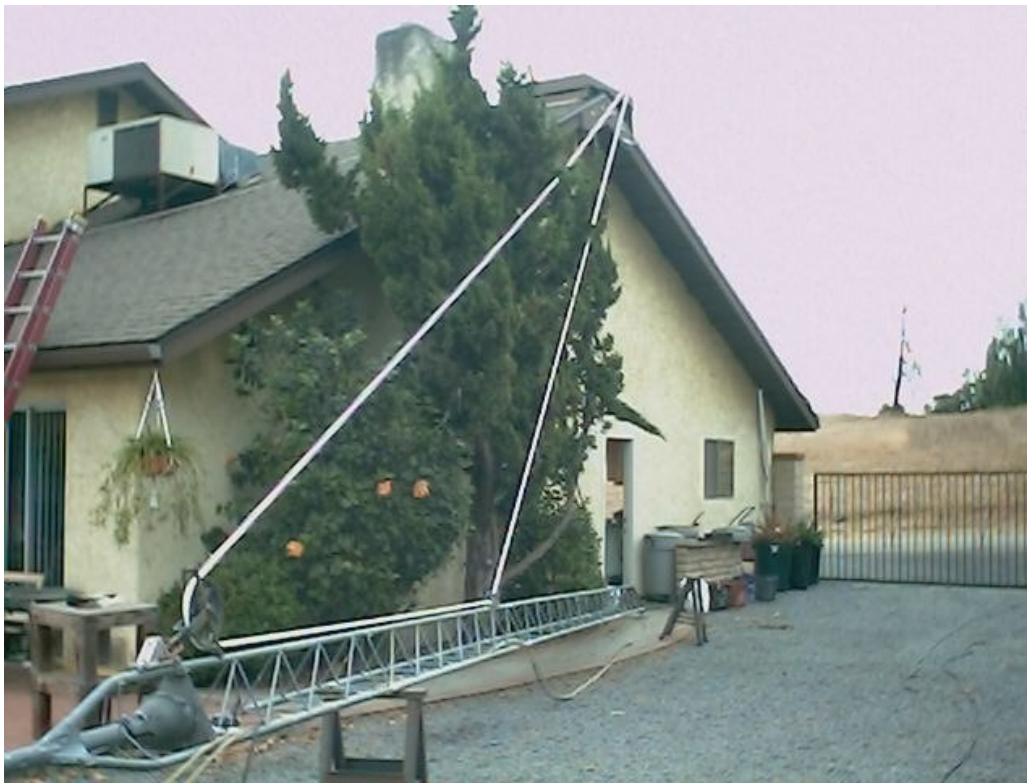
You can see how this works. There is a double pulley (2 grooves side by side) on the roof.
