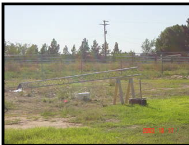
After getting ten feet up the section is laid over and another 20 feet added.
