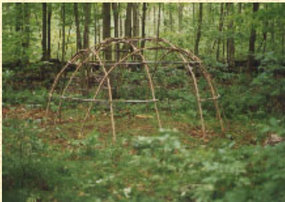
The completed sapling frame of my wigwam in the northeastern connecticut woods. The poles are made of sassafrass, the hoops are made of sweet birch.
