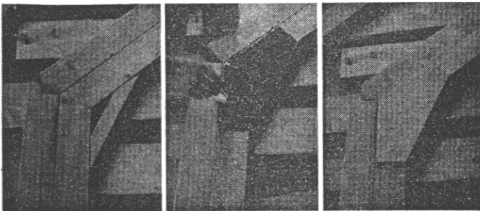
A rigid frame formed in a jig with plywood gussets being glued and nailed over the joints. Note the filler block which may be cut from a 2" x 2" (shown) or 2" x 4" member. Fourpenny nails secure the gussets until the glue dries.
