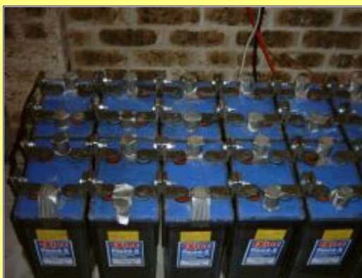
Half of the battery bank.
