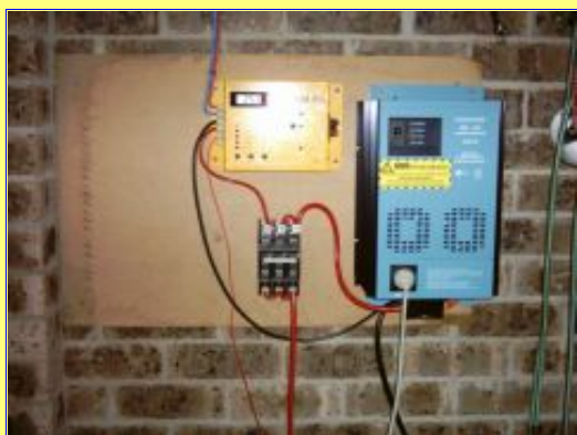
The switchboard consists of a charge controller (yellow box), inverter (blue box) and a Real Big Switch.
