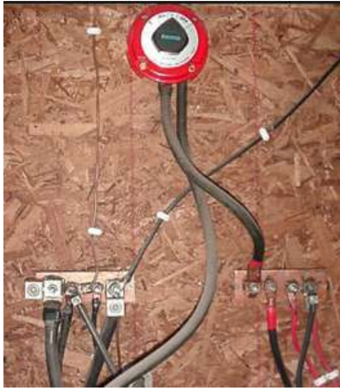
My buss bars and main power switch
