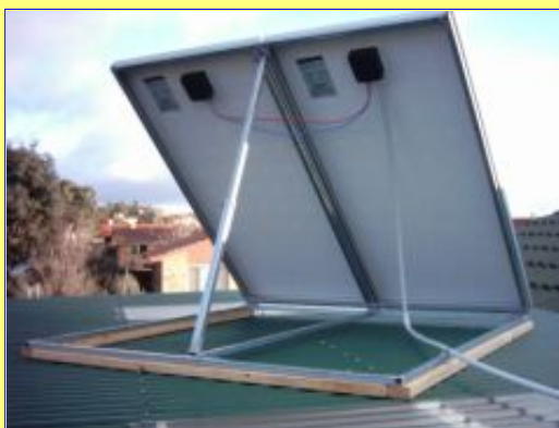
The rear of the solar panels, showing my homebrew rack. The timber is to prevent scratches on the colourbond roofing.
