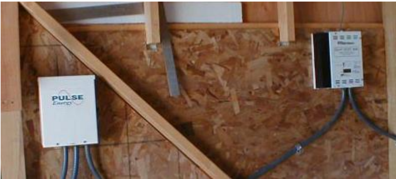
The PV combiner box and solar boost 3048 charge controller. These carry 48volts from the PV panels.
