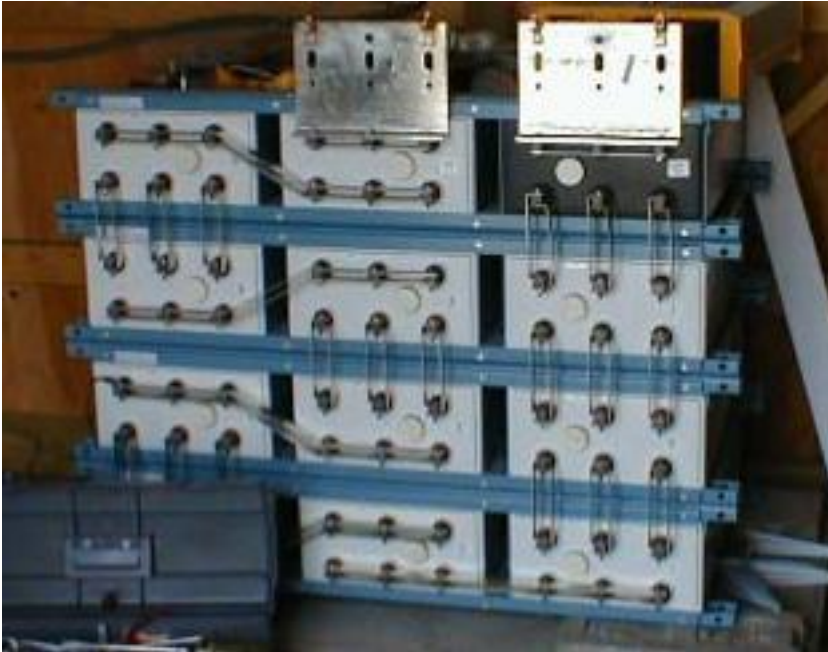
The 24 volt battery bank. Wieghing in at over 3000 lbs. These are lead cadmium telco UPS batteries. They are not meant to cycle more than 15% from full charge.
