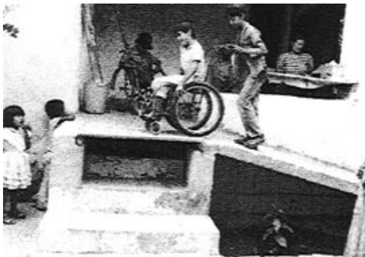
This ramp in a Mexican village clinic was built in a very limited space. The board over the steps lifts out of the way, so that people can use the steps when the ramp is not needed.
