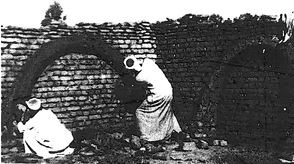
FIGURE 5. Two masons are seen applying the mud guide ring which will tie the vault to the end wall. The end wall has been built above the limits of the proposed vault and has had sufficient time to dry and reach its maximum stability. It is now ready to receive the thrust of the vault. Before Gourna Village was started the masons would make this mud ring guide by guess work and by eye. Dr. Hassan Fathy speeded up construction time by making a wood template in the shape of the under side of the vault and using this template as a guide for this mud ring. A more uniform vault was the result, plus a saving in time. In addition, at New Gourna, two masons, rather than one, work on the vault. One helper can supply material for both masons.
