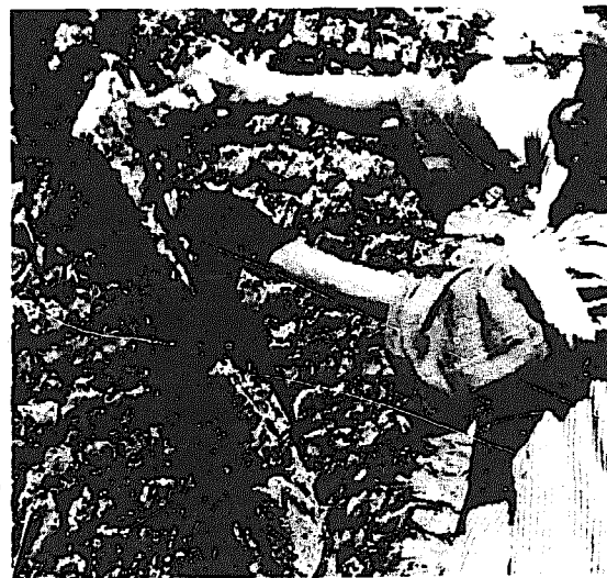
FIGURE 12. The mason is placing the last brick in the fifth course. The cant of the courses is now well established.
